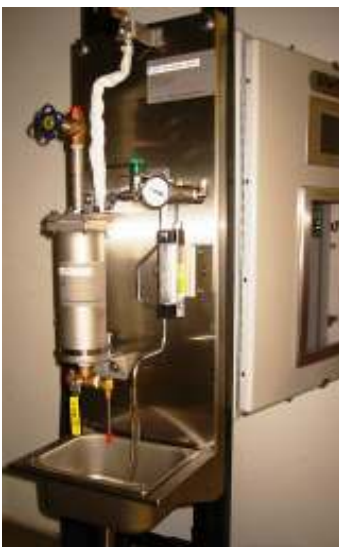
(Heat Exchanger and Sample-Conditioner System)
